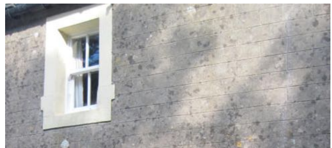
Smooth render lined out to imitate stonework
